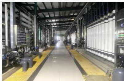
Boiler Feedwater Treatment System Project of Thermal Power Plant for Yihai Jiali (Fuyu) Energy Co., Ltd.
