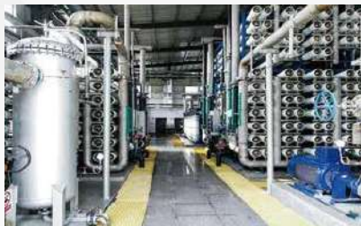
Woniushan Waterwork of Yantai Economic & Technological Development Zone Tap Water Co., Ltd.
