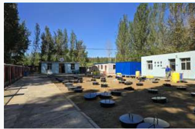
Dongguan Sewage Treatment Plant Project in Beipiao City
