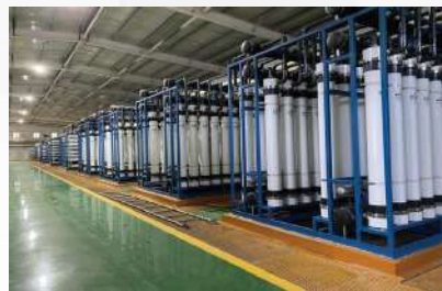
Demineralized Water Treatment System for 50,000-ton/year Dodecanedioic Acid Project of Ningxia Hengli Biomaterials New Materials Co., Ltd.
