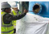
Filter media replacement
