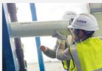
Membrane element installation & commissioning
