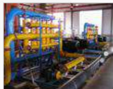
Seawater Desalination Unit
