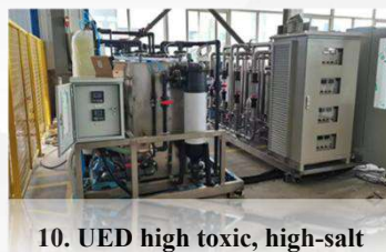
10. UED high toxic, high-salt & high-concentration wastewater treatment unit
